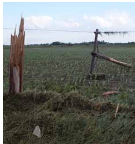
Tornados and strong winds splintered poles and left grass hanging from the conductor in some areas.
