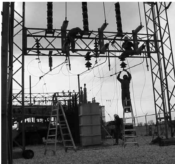
Smart grid technology will give utilities more information about the way the electric system is working. One of the advantages is detecting problems before they become outages.
