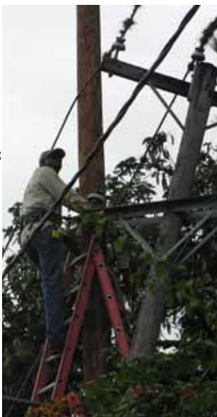
Linemen in Haiti usually use ladders to access line hardware instead of bucket trucks. The job is a dangerous one -- with fewer safety rules in place than in the U.S. Fourteen EdH linemen lost their lives on the job in 2010.
