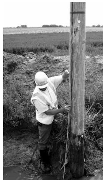
A Dawson PPD lineman measures the amount of soil removed near this pole. Removing soil weakens the power line, increasing the chance that strong winds could topple the poles.
