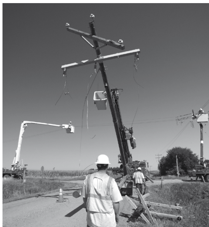
ABOVE: Crossarms and insulators are added to the new pole before it is set in the ground. As the new pole is set, the linemen will remove hardware from the old pole so hardware can be salvaged and reused. (Photos: M Holscher Banzhaf)
